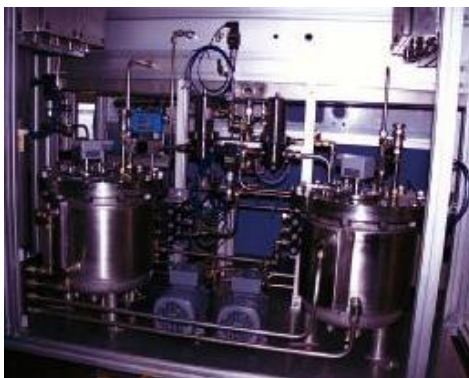
Blick in den Hydraulikraum
